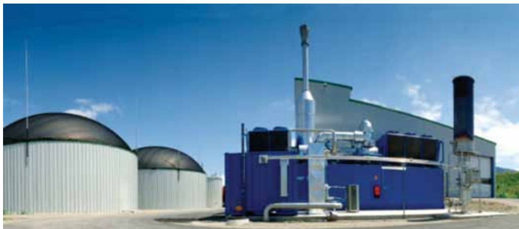
Figure 10.16 A modern biogas plant [15]
